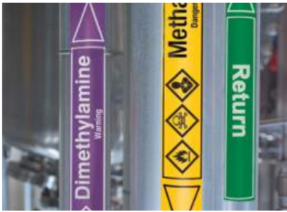
Pipe & valve marking
