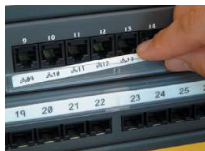
Punch block & patch panel labels
